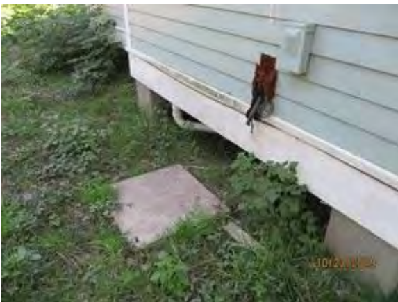
Missing AC Unit
