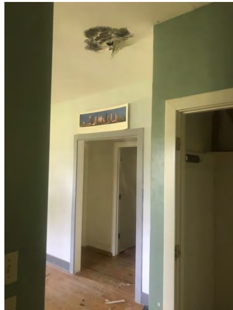
Damage in ceiling (family room)
